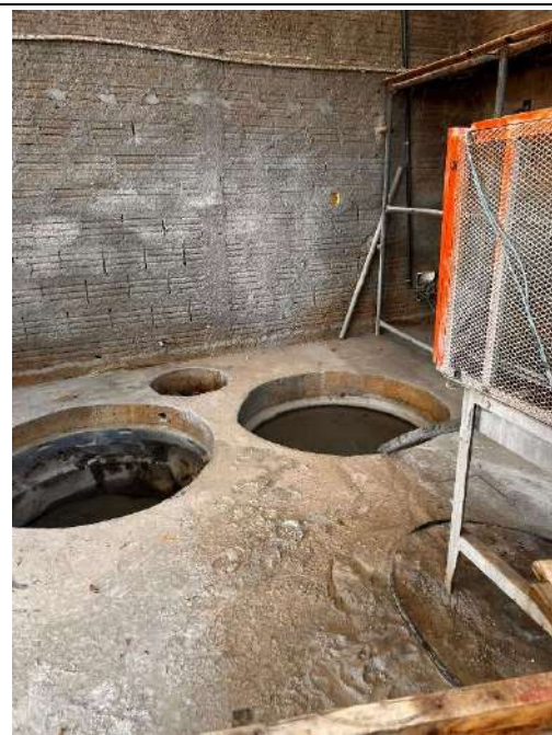
Drill core cutting saw sediment settling tank.
