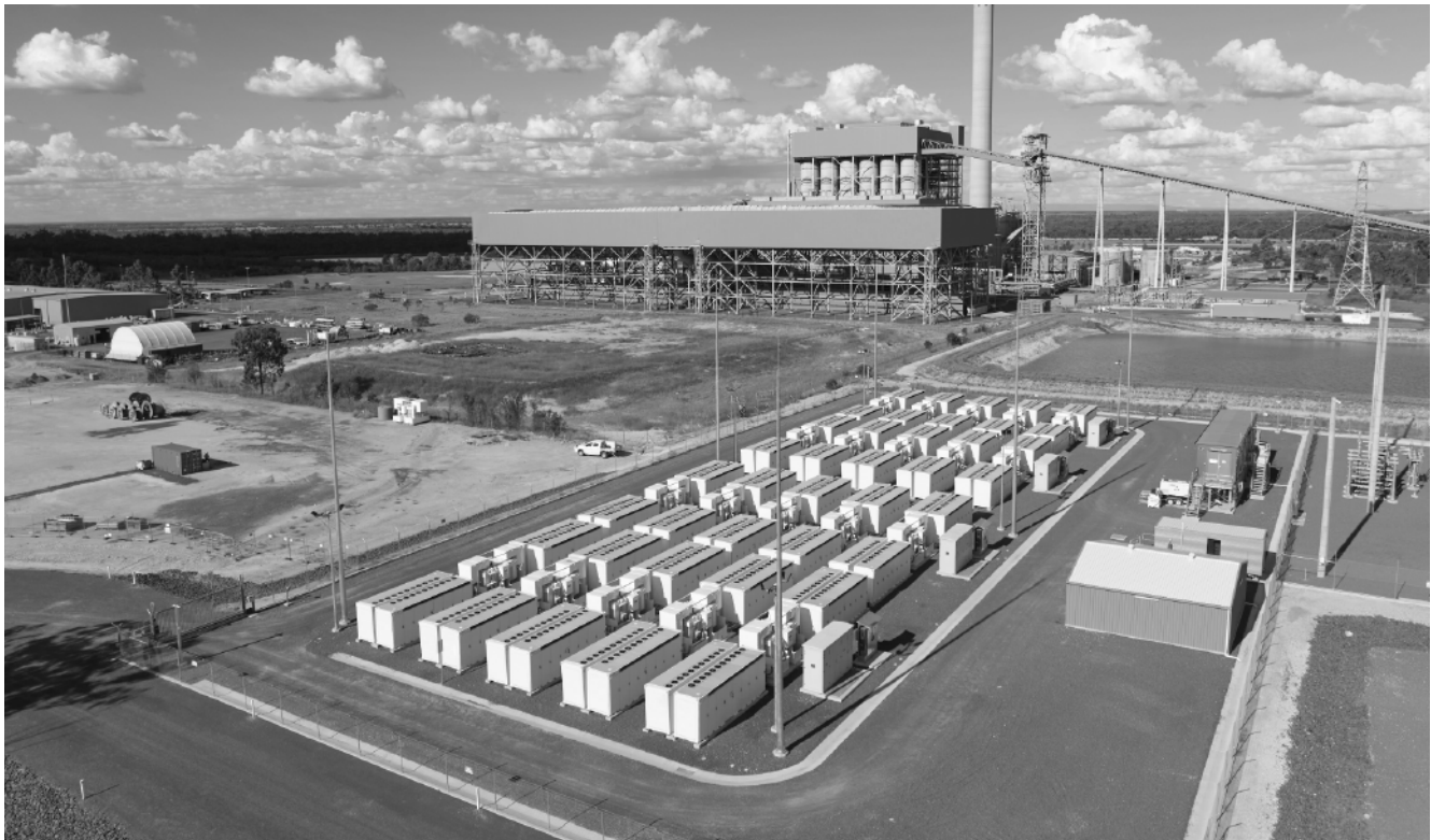
Construction and commissioning of the Chinchilla Battery was completed this year, and it began commercial operations in July 2024.
