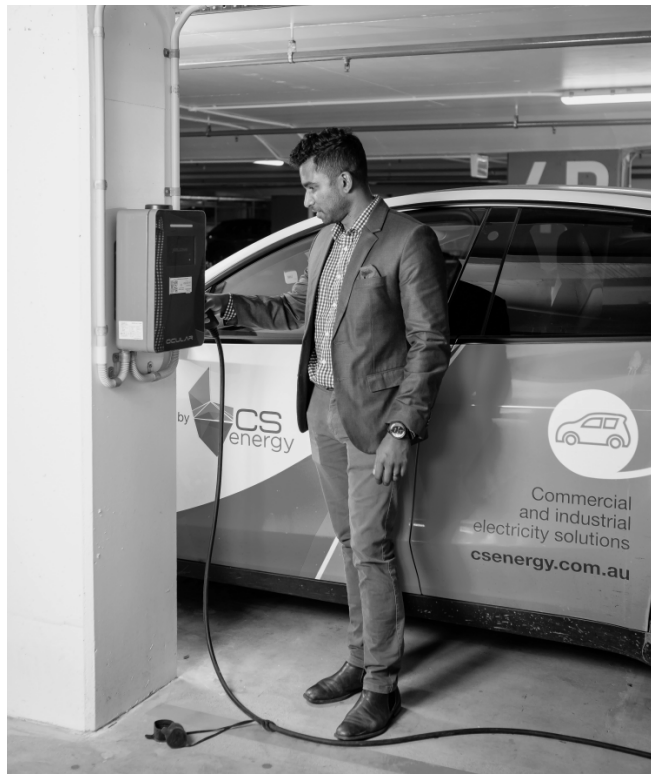
CS Energy has installed EV chargers at 260 customer sites to date, as well as at two of our sites. Digital Products and Platforms Manager Lahiru Wimalasuriya is pictured using one of the chargers at our Brisbane office.
