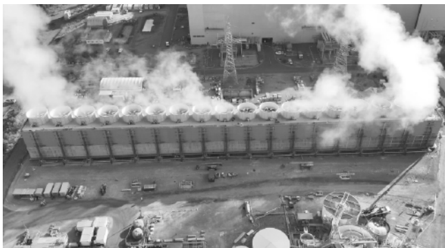
New C3 cooling tower in operation.
