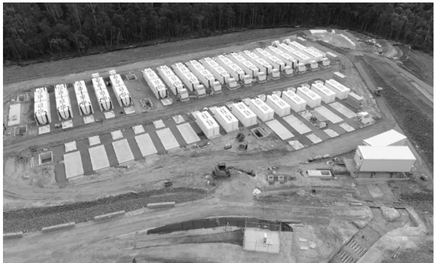
The Greenbank Battery will be CS Energy's second battery project and is located next to Powerlink Queensland's Greenbank Substation. This photo shows construction progress as of end of FY2024.
