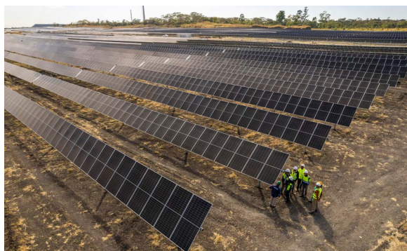
35MW solar photovoltaic (PV) installation at Zimplats
