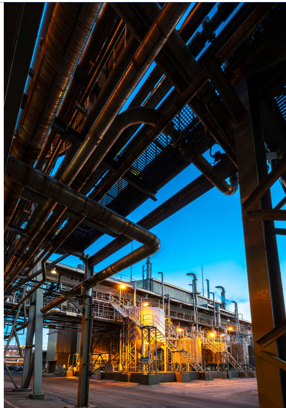
The nickel recovery plant at Impala Refineries, Springs
