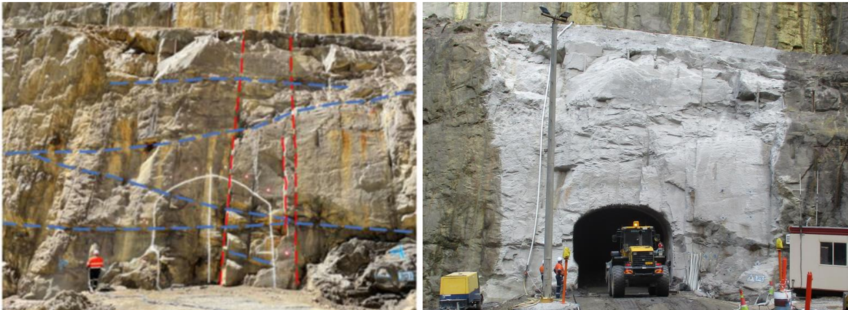
Figure 24: Mapping of the dominant geotechnical features in the exploration decline portal face (left) and the established 900 exploration decline portal (right)
