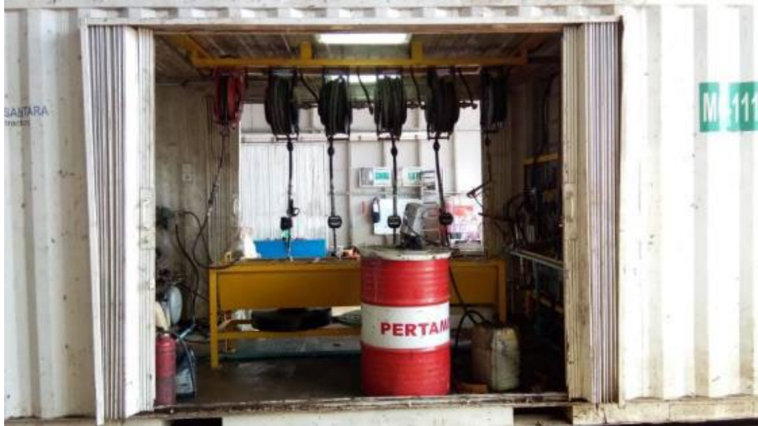
Figure 30 HV Workshop Lube container
