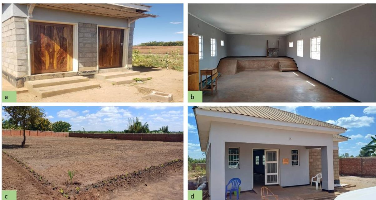
Figures 4a-4d: Upgrades to the Malingunde Community Centre sponsored and supervised by NGX.
