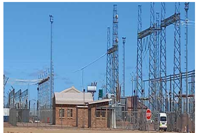
Photo 8: Newly built Nieuwehoop sub-station (near Kenhardt).
