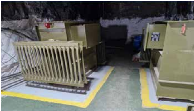
Photo 4: Underground 178m Level Electrical Sub-station.
