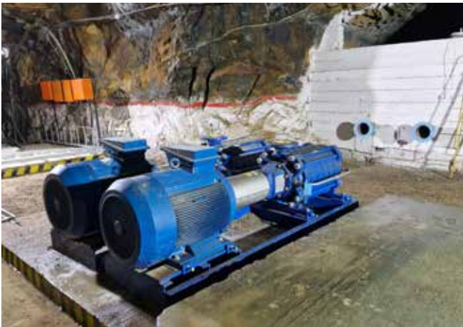
Photo 3: Underground 178m Level Multi-Stage Pumps.
