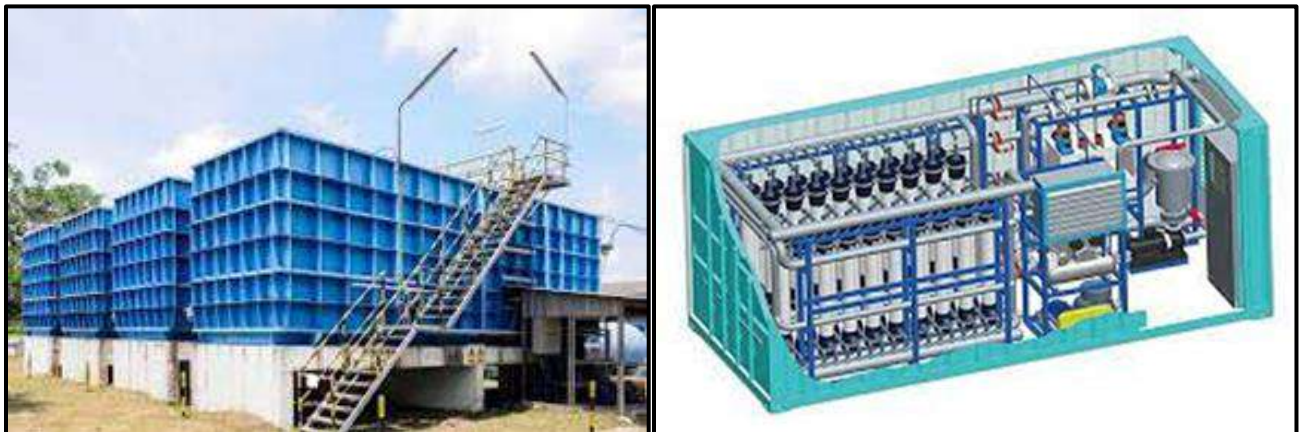
Figure 18-3 Containerized wastewater treatment plant and containerized potable water treatment
