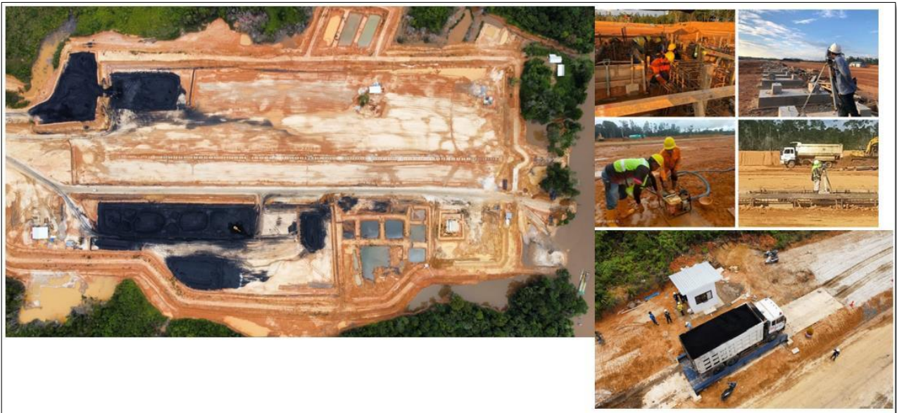
Jetty Batu Tuhup Development Progress (Weight bridge and foundation has been in place)
