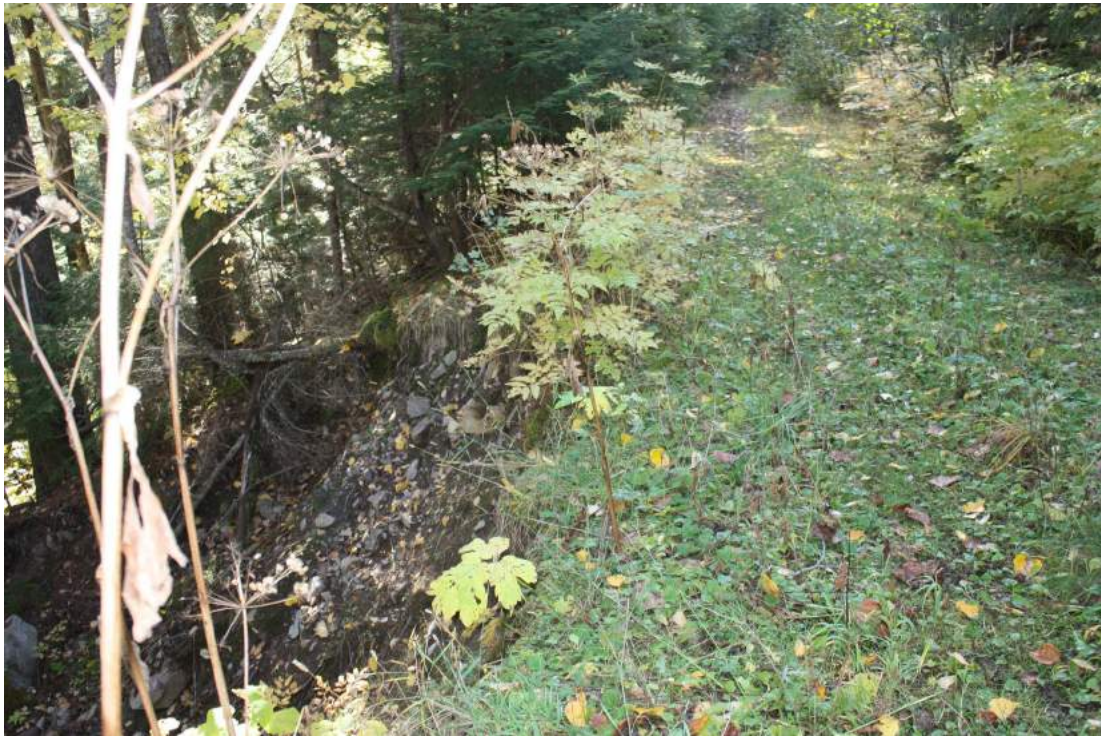
Washouts along the road
