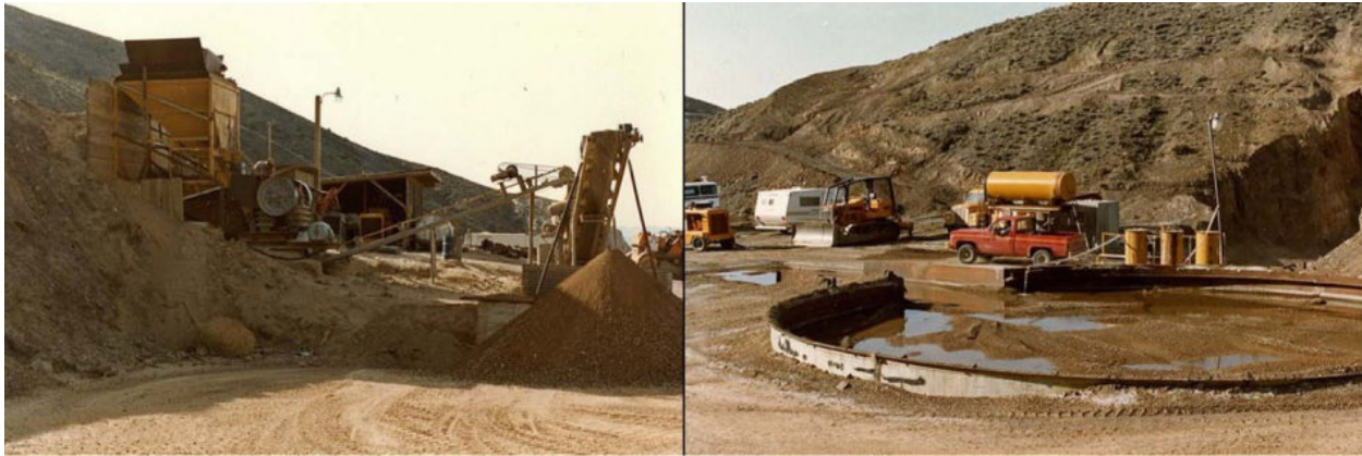
Figure 6-1: Fisk Crusher and Vat Leach Operation
