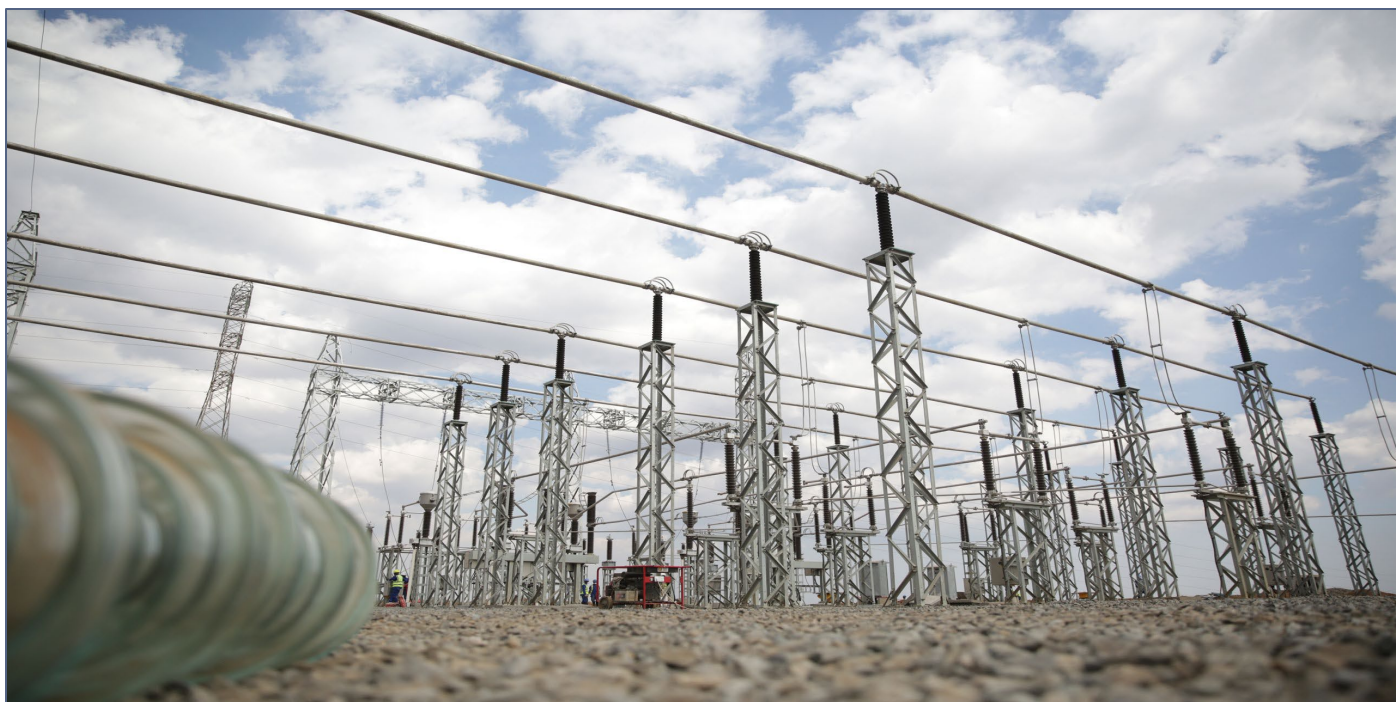
Figure 19: Nkhoma substation has capacity for connection to the Kasiya operation (Source: Millenium Challenge Corporation, USA)
