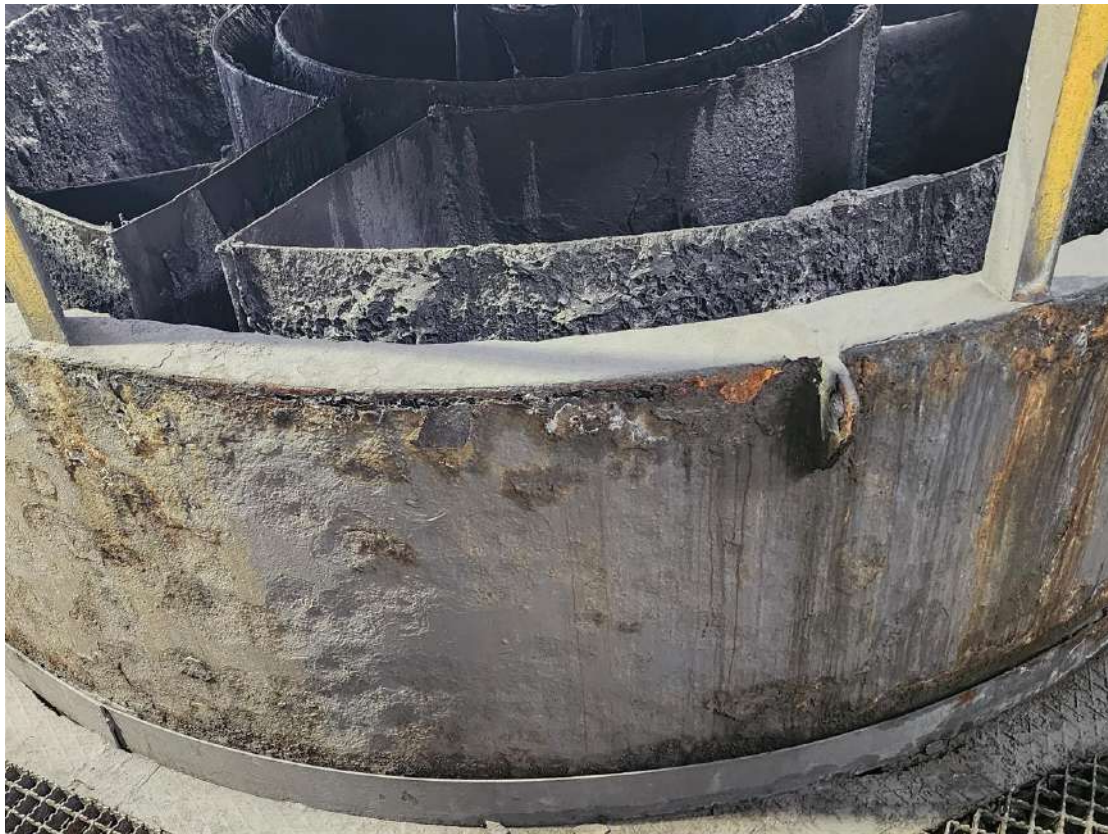
Figure 17.10 Corrosion around the top of flotation columns; requiring replacement
