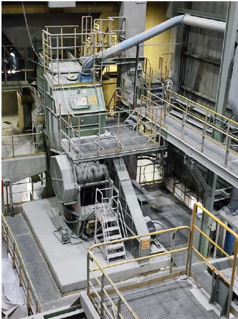
Figure 17.5 Primary crusher installation
