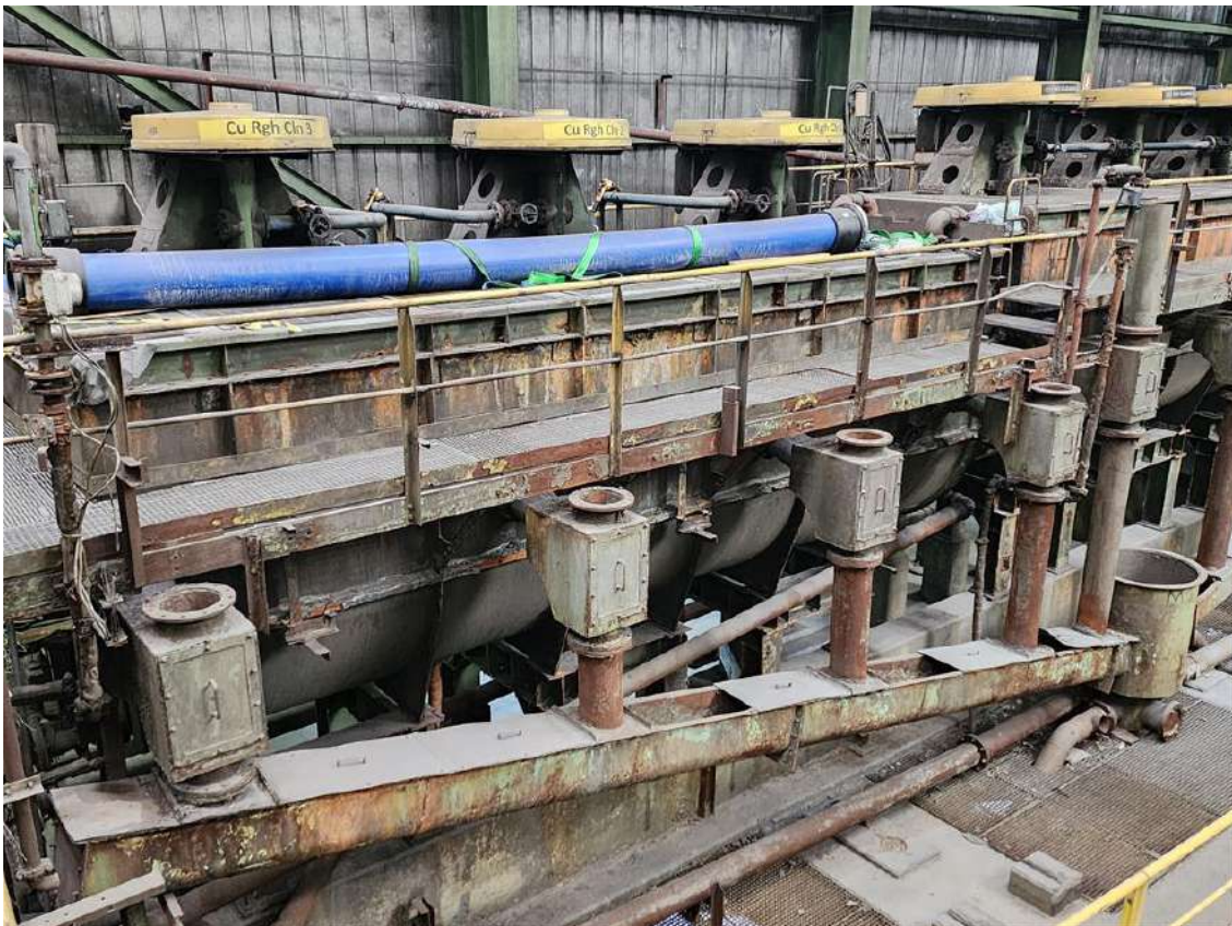
Figure 17.9 Cu rougher cleaner cells requiring replacement
